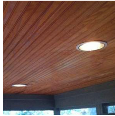
① SOFFIT LIGHTING
