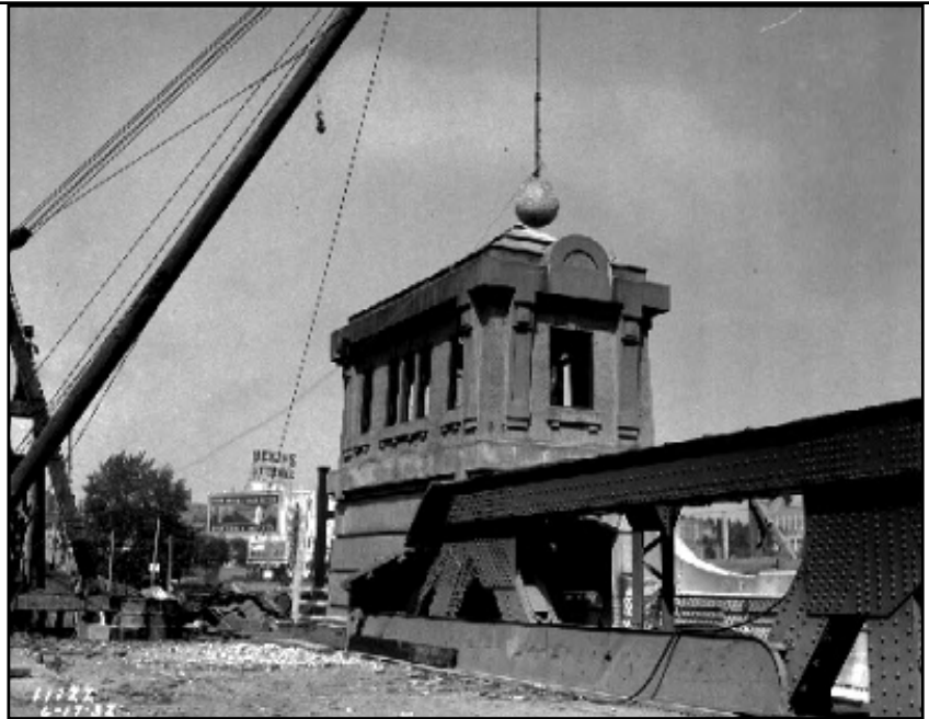
The wrecking ball is poised above one of the four original towers of the University Bridge just before it is about to be demolished in 1932 to make way for the bridge expansion. Photo was taken from the bridge deck looking northeast. Courtesy of Seattle Municipal Archives, No. 5811.
