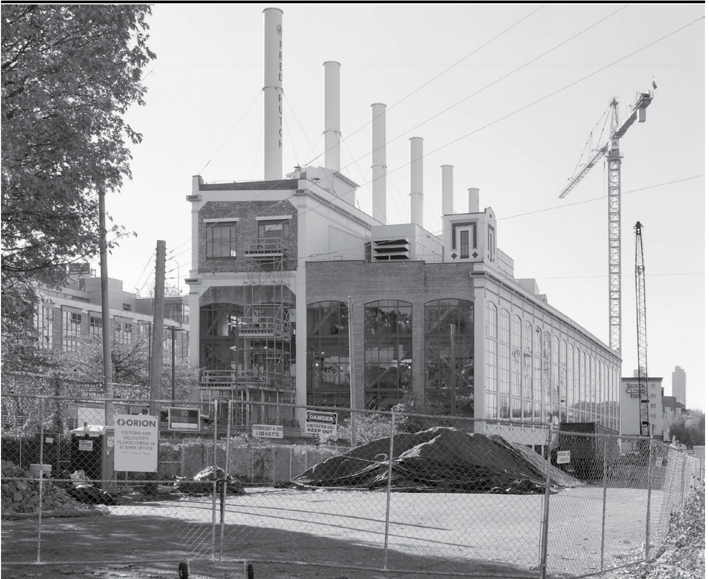
The Borders of Eastlake: The south border is usually considered to be around the historic Lake Union Steam Plant building, seen here with its current updating construction project under way and the cranes for the Fairview bridge replacement in the background. Read more on the newsletter's border project pages 3 and 11.
