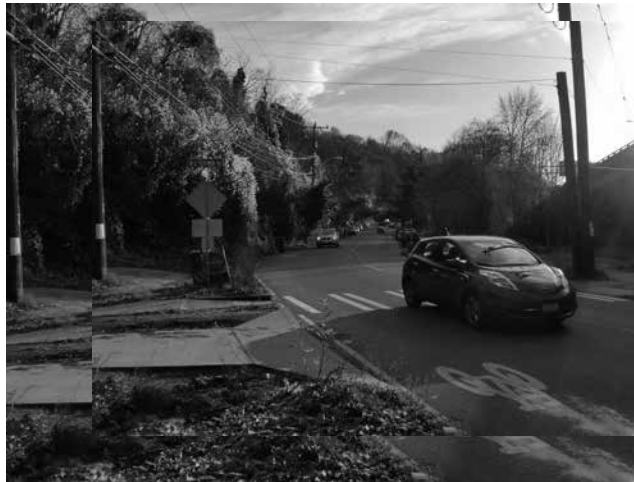
Where the sidewalk ends. Another missing link, this one is the lack of sidewalk on Lakeview Avenue. between Howe and Blaine staircases.
