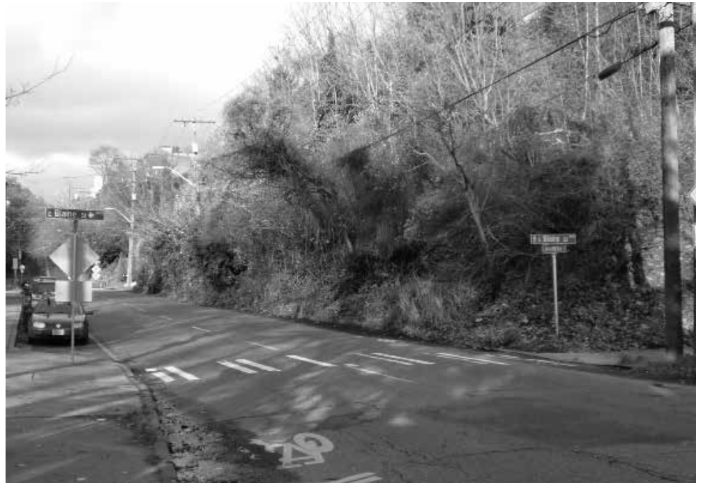
Lakeview Blvd. between the Blaine and Howe Street stairs lacks a sidewalk and a retaining wall. Note how sliding into the street has covered the curb, posing special dangers for cyclists and pedestrians.
